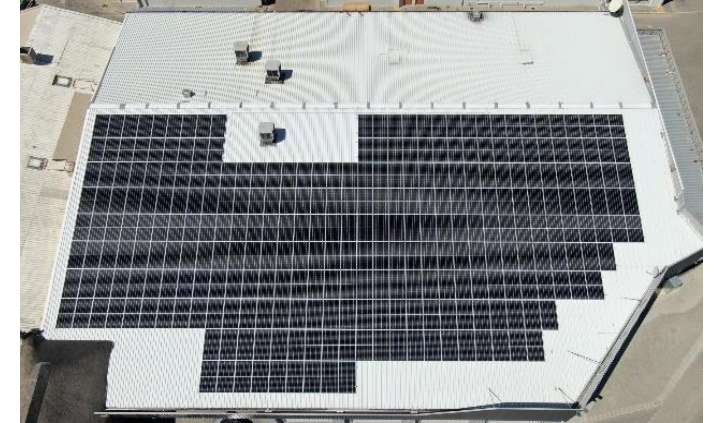
Food Market, Northern Cape, SA 125 kWp (2020)
