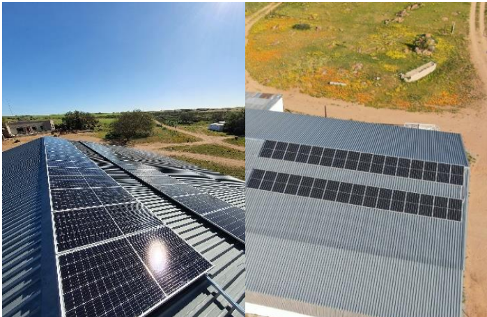
Farm House, Northern Cape, SA 6.2 kWp & ESS (2020)
