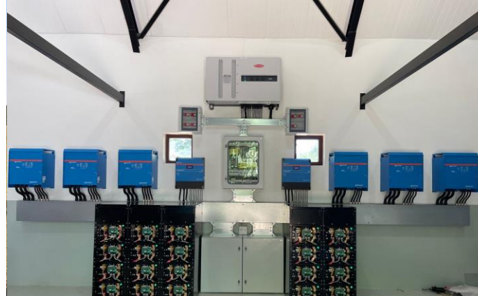
Wine Farm, SA 80 kWp, 357.5 kWh (2022)
